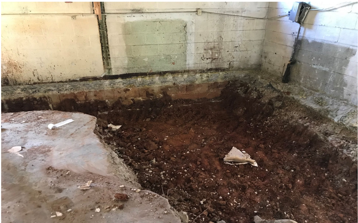
Figure 25: Backfill of clean soil after removal of impacted soil below building floor slab
