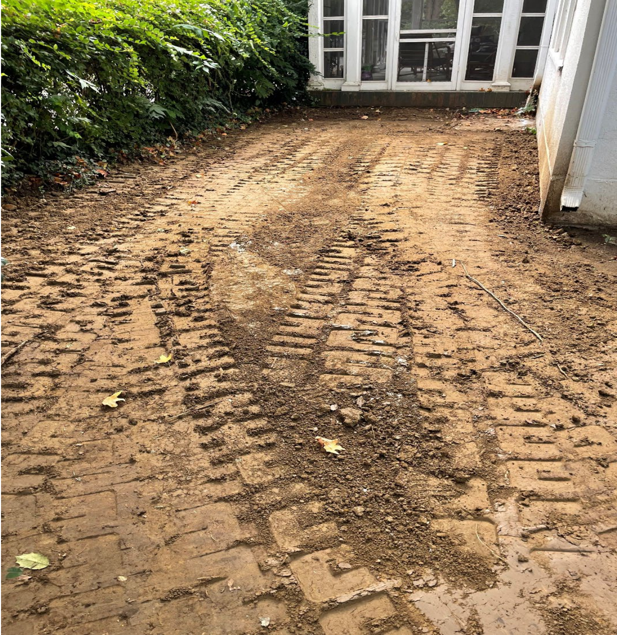
Figure 24: Photograph of Wright Property Backyard after removal of impacts from the 2020 release. Soil backfill prior to placement of sod
