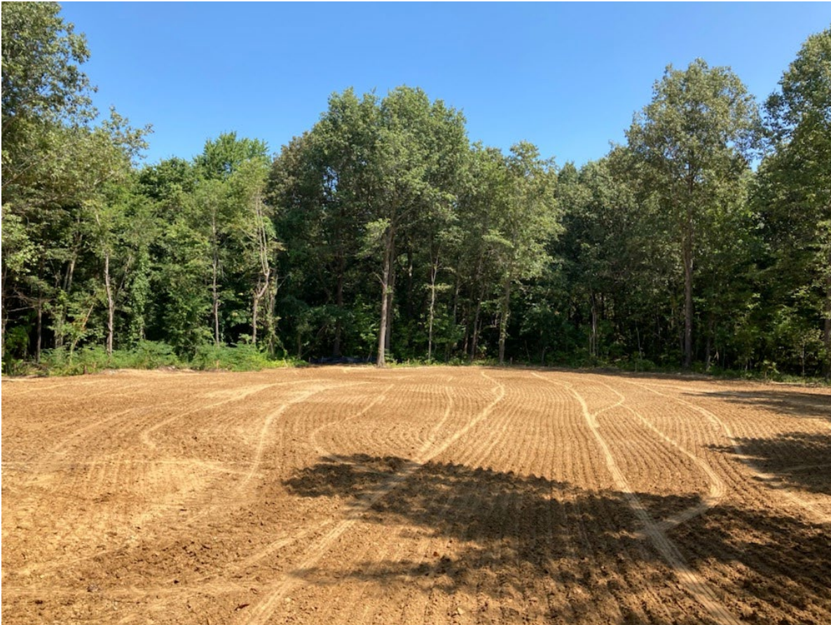
Figure 20: July 2021- View of the above area after it was backfilled with clean soil and seeded.
