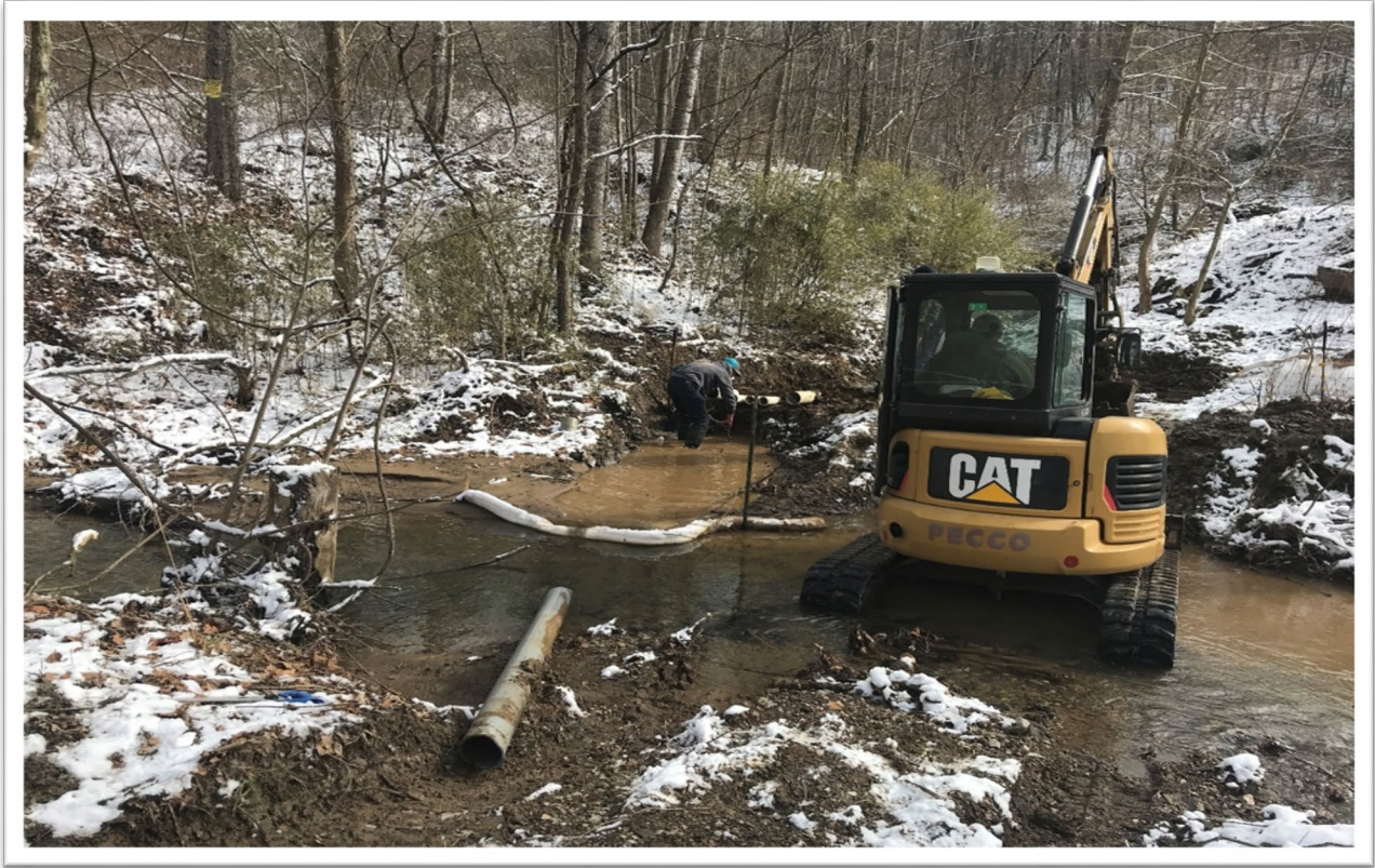
Figure 10: RN Sparks Crude Oil Spill, construction of emergency underflow dam for product collection.
