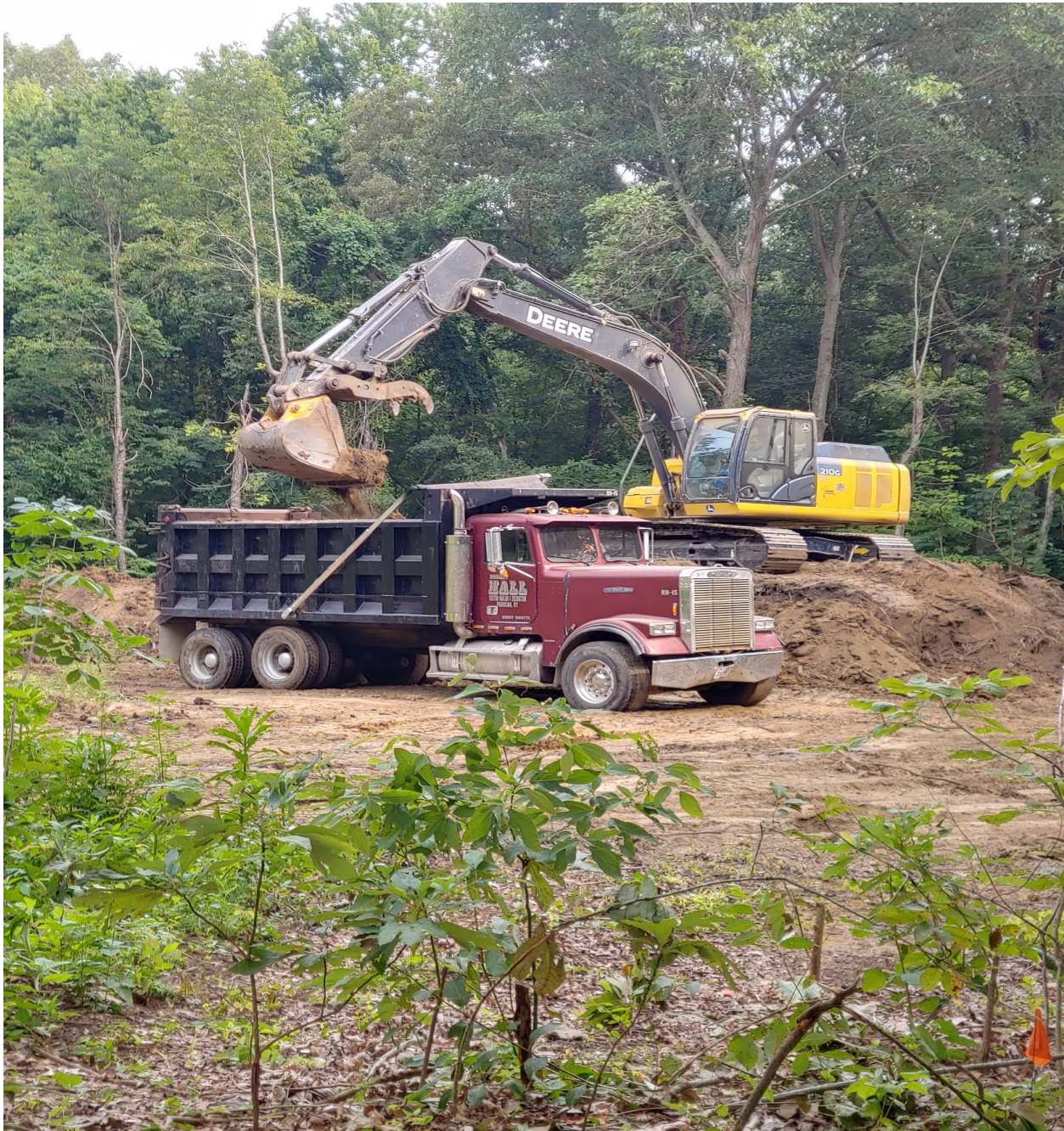
Figure 18: July 2021- View of the contaminated soil loaded for disposal at a contained landfill.
